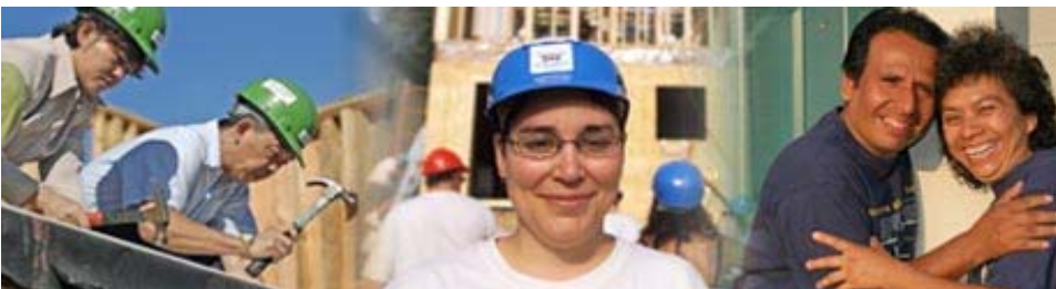
Try on the smile that comes from laying a foundation with kids from Habitat and its soul-sister – Vista's AmeriCore .
